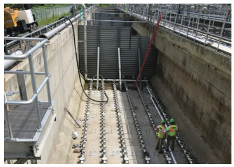
Hydraulic capacity and treatment improvements were completed in 2020 to increase plant capacity and provide enhanced wastewater treatment prior to discharge into the Lackawanna River. In 2021 and 2022, the company rebuilt the headworks facility, removing the chlorine gas disinfection process and rebuilding the facility’s sludge handling process.
