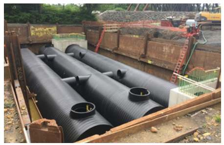
A 120,000-gallon equalization system was installed to substantially reduce combined sewer overflows into the Lackawanna River. This is one of over 60 CSO reduction projects completed as part of the LTCP.
